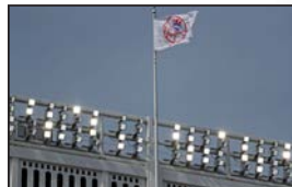
The Yankees installed new LED lighting prior to the 2016 season, reducing Yankee Stadium's carbon footprint.
